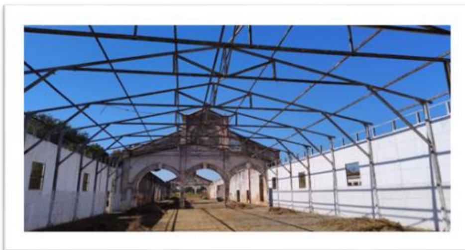
Figure 3 – Remnant of the old welding workshop
